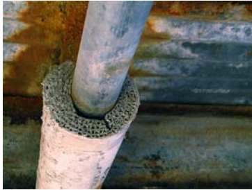
Asbestos pipe insulation
